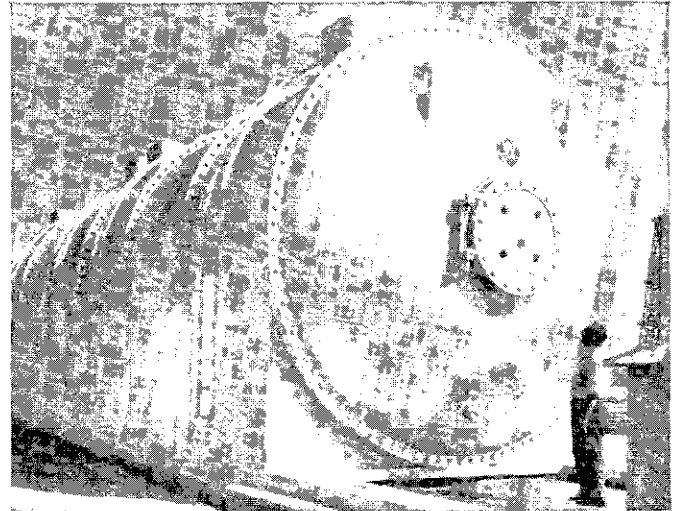
Fig. 5—Hydrogen-cooled frequency changer set installed on the system of the City of Los Angeles, 60 000 kva; 600 rpm; 50 cycle—11 500 volts; 60 cycles—13 200 volts.
