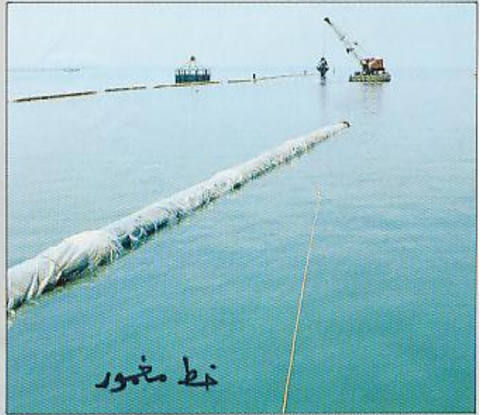
Sewage pipeline (Submerged piping)
