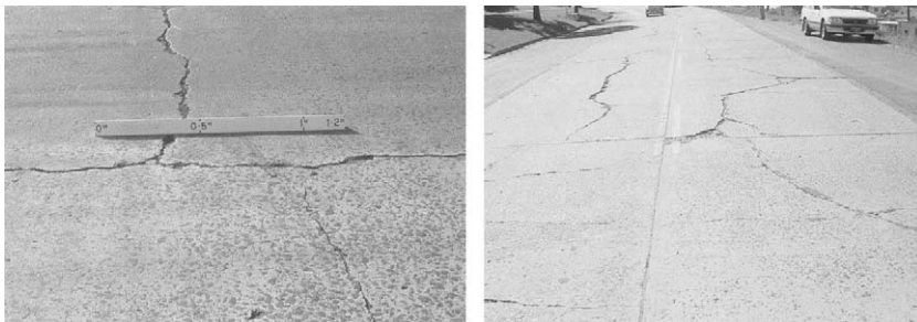
FIGURE 19.32 Block cracks in rigid pavements (Source: Austroads, 1987).
