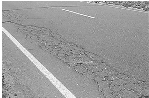
FIGURE 8.5 Advanced stage of fatigue cracking.
