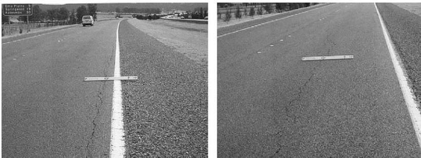
FIGURE 19.10 Longitudinal cracks in flexible pavements (Source: Austroads, 1987).
