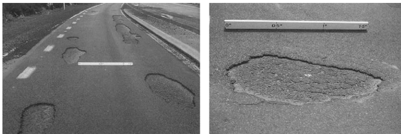
FIGURE 19.17 Delamination in flexible pavements (Source: Austroads, 1987).
