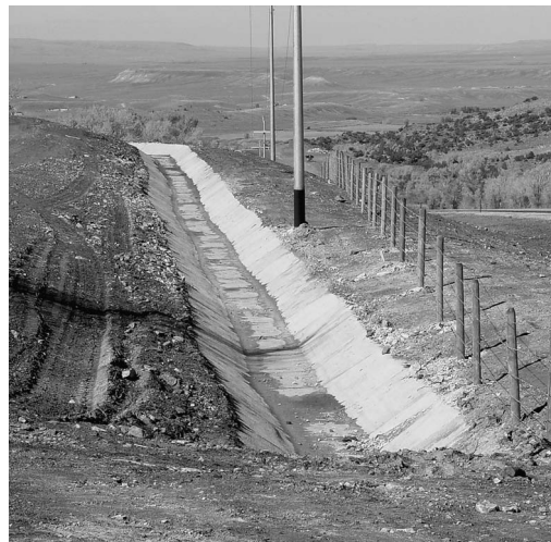
FIGURE 13.6 Concrete linked ditch.
