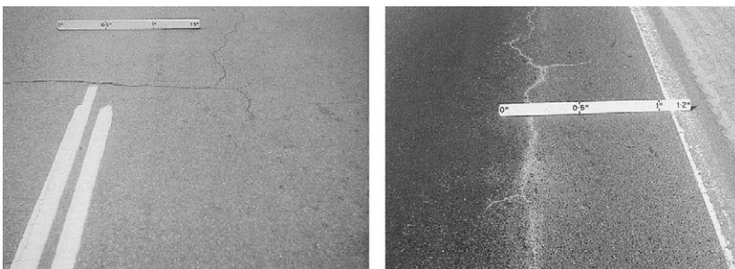
FIGURE 19.15 Meandering cracks in flexible pavements (Source: Austroads, 1987).
