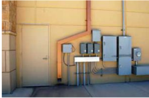
Electrical panel locations in lease space
