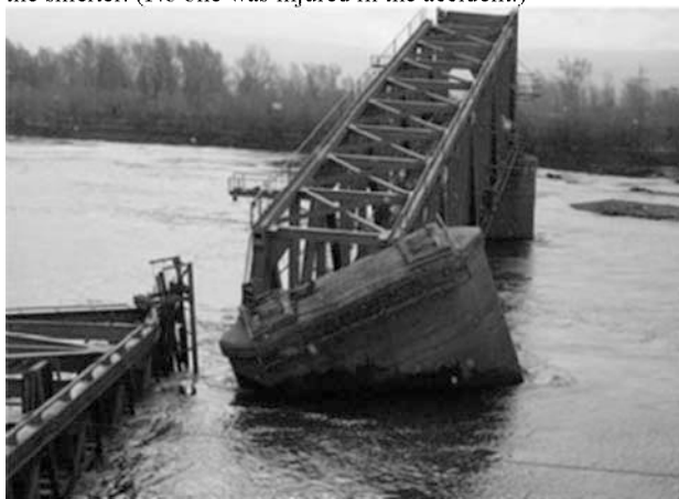
Figure 1. The collapsed bridge
