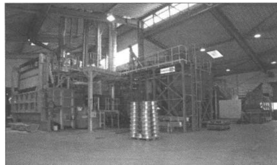
(Swarf Plant equipped with charge hopper, pre-treatment high speed co-flow dryer)
