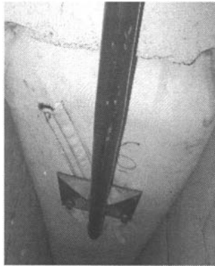
Figure 3: Inflatible gate in position in the port
