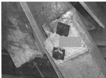
Figure 12 – Example of damaged end riser.
