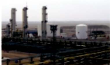
Water purification station
