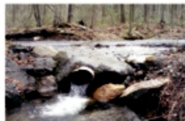
Discharging sewage in canals
