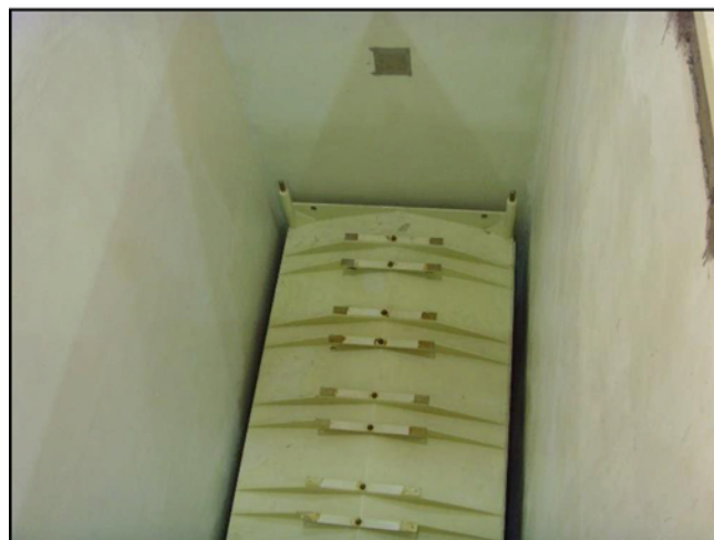
Figure 2 Stainless steel vertical casting pit built in 2012 coated with Wise Chem E-115
