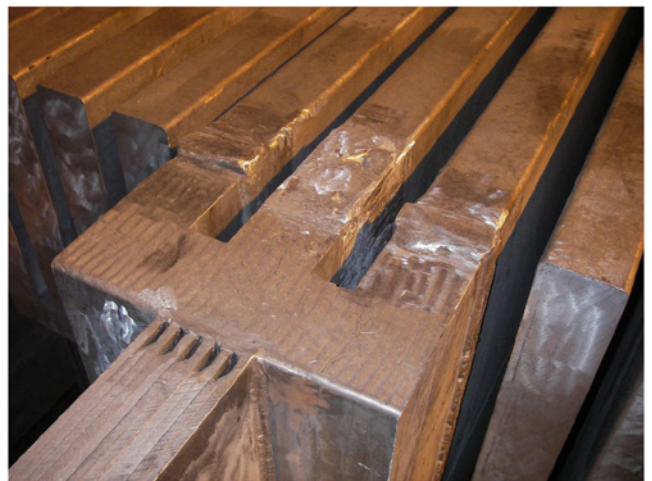
Figure 12: Example of a change in the bus bar configuration of a smelter in operation
