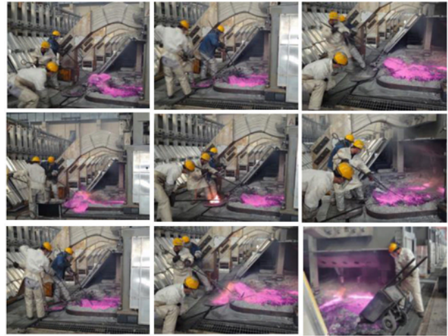
Figure 2: A series of snap shots of manual anode cavity cleaning process (Procedure I)
