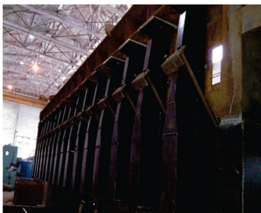
Figure 11 160kA Pre-stressed cell shell of Chalco Guangxi Smelter
