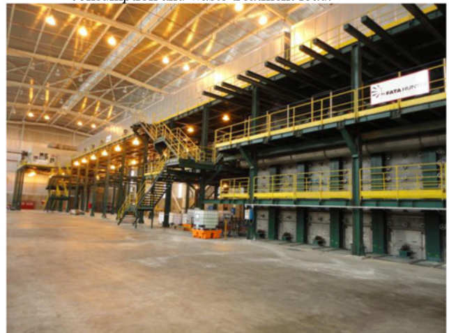
Figure 5. Vertical Wet Section of the Coil Coating Line.
