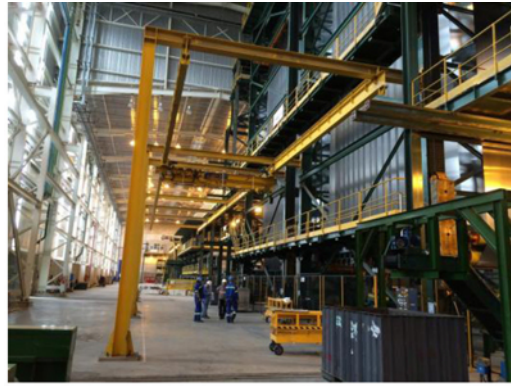
Figure 10. View of the entry section and of the crane structure for replacing rolls in tower.
