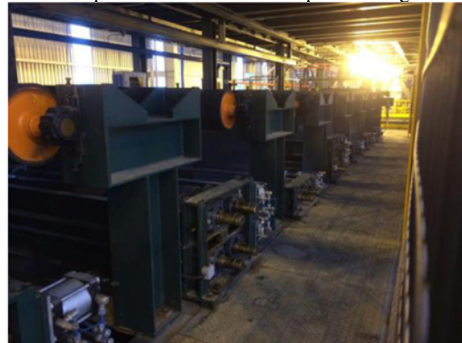
Figure 11. View of the Wet Section of the Coil Coating Line.
