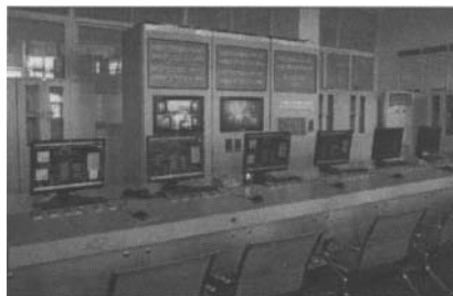
Fig.5 Control room of Aohai Carbon's power station
