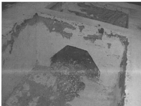
Figure 2. DOE-1 Furnace during a cold cleaning after ~1 year of service.
