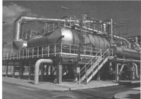
Figure 6 – A typical MED plant installation
