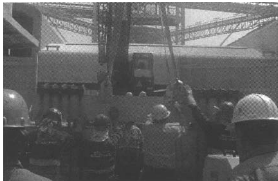
Figure 17: Closure of Line 1 South End Temporary Switch
