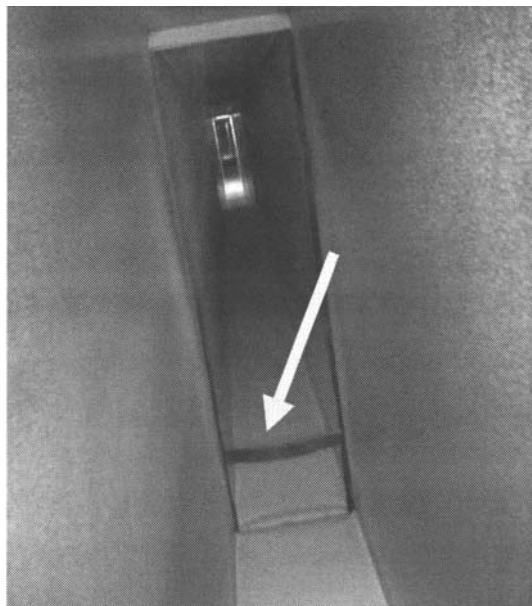
Figure 6: Gasket that is installed upside down
