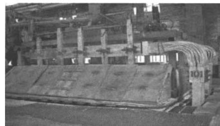
Fig.6 80 kA prebaked cell retrofitted from Soederberg cell
