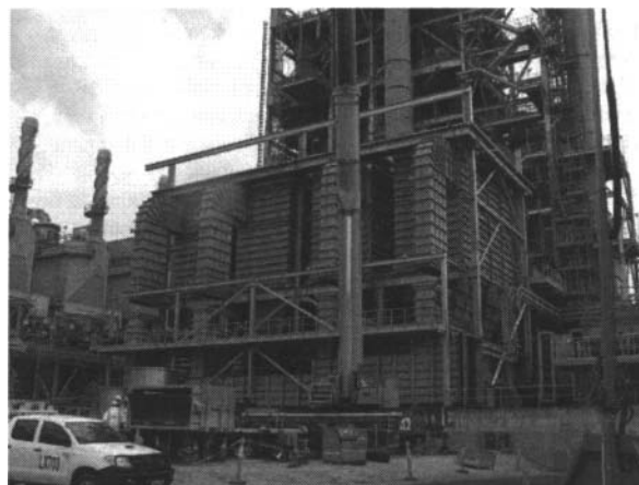
Figure 12. FabriClean filter installation at Worsley
