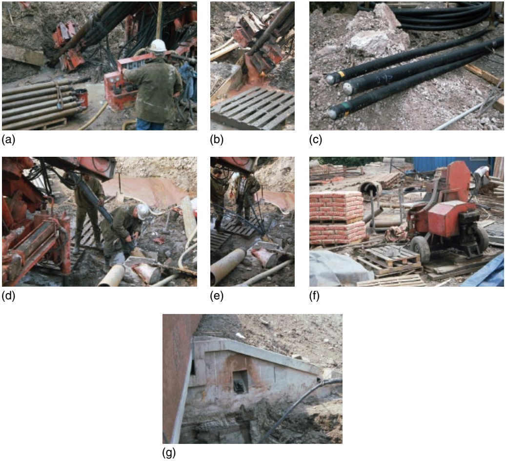
Figure 15.3 Ground anchor installation. (a) Drilling (Class C 2 3 3), (b) Pressure test, (c) Tendons, (d) Taping injection pipe to tendon, (e) Tendon strands, (f) Cement and grout pump and (g) Anchor head.
