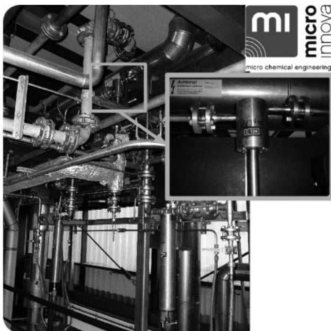
Figure 12.3 StarLam 3000 in production surroundings [21].
