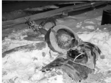
Failure of fire hydrant
