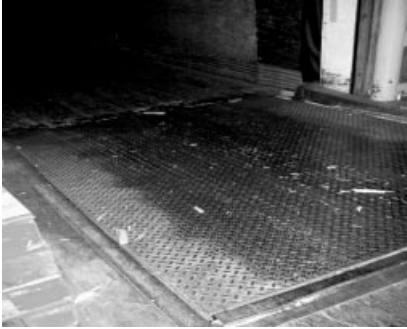
Figure 14.2 Dock leveler between truck trailer and concrete loading dock.
