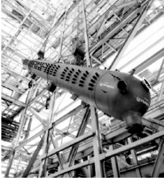
Figure 10.4 A typical steam drum being lifted into place in a boiler during construction (Babcock and Wilcox).
