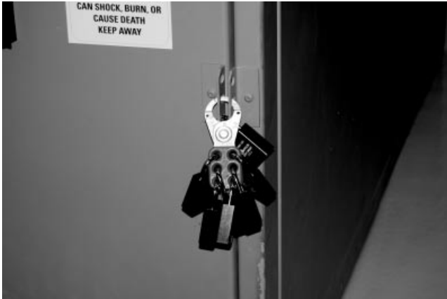
Figure 7.4 Multiple locks used to lockout a switch gear cabinet.
