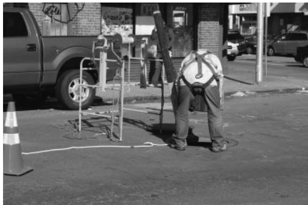
Figure 7.2 Work in a manhole. Telecommunications and electrical utility work performed in manholes is considered work in a confined space.
