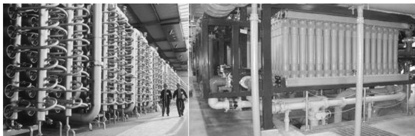
Figure 4.15. Industrial plant for desalination of seawater
