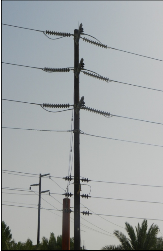
115 kV &amp; 13.8 kV
