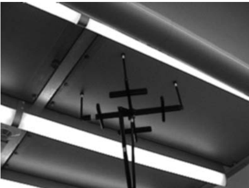
FIGURE 2 Proper use of tube array to determine filter face velocity.
