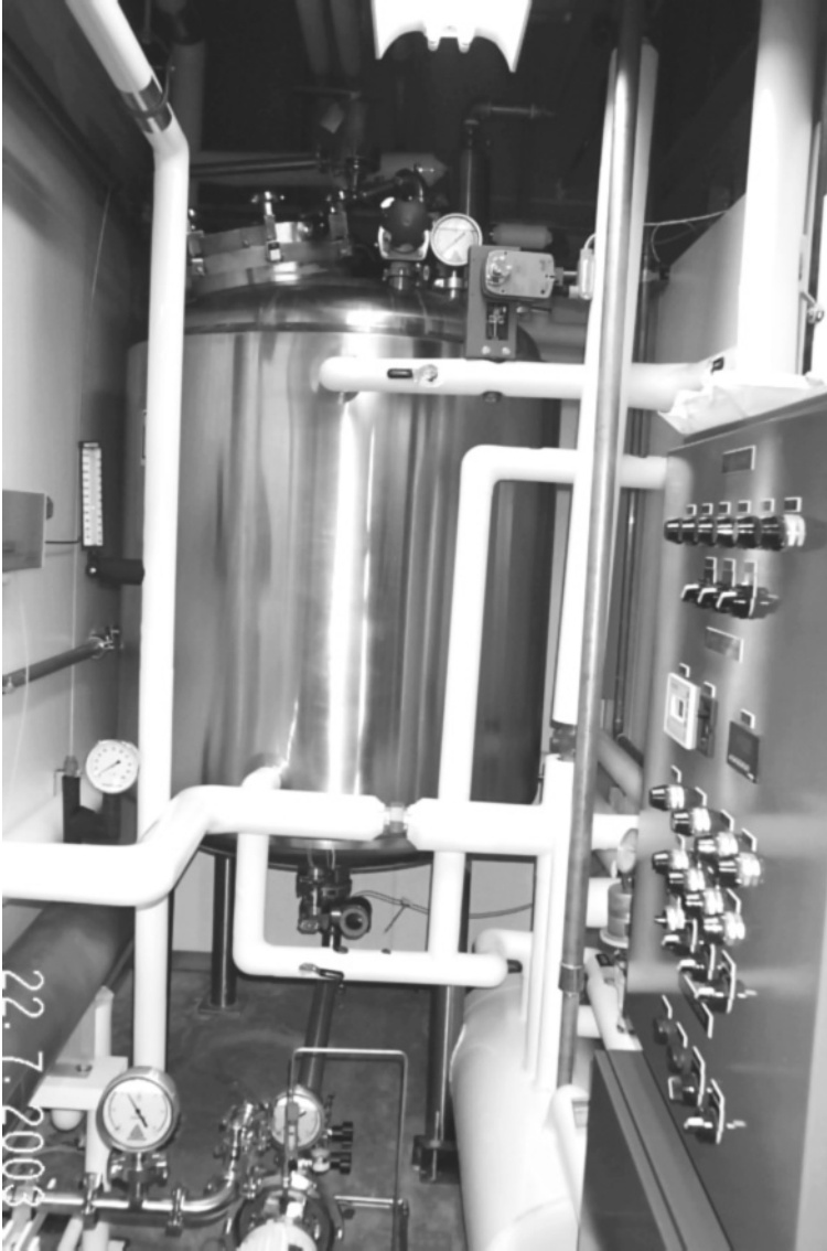
FIGURE 3 WFI storage tank and control panels.
