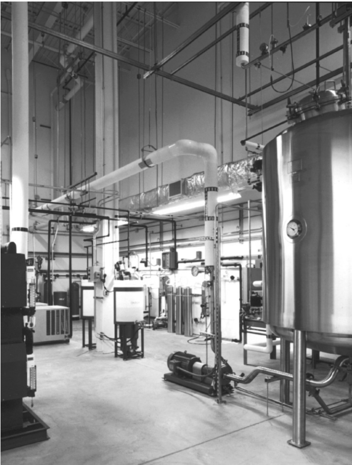
FIGURE 2 Water plant with holding tank.
