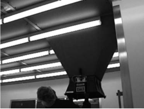
FIGURE 1 Proper application of a flow hood to determine filter volume.
