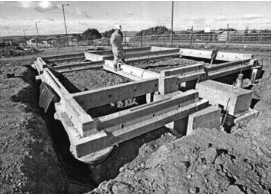
Figure 8.6 Piling system to isolate houses from heave of slag – courtesy of Roger Bullivant Ltd
