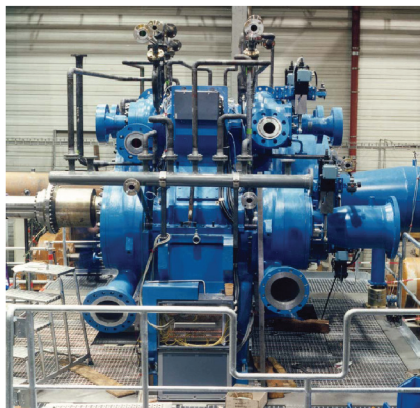
Figure 5: 125 tonne/hr RG080/8 MAN Turbo compressor at the Dakota Gasification Company providing CO 2 to the enhanced oil recovery fields at Weyburn and Midale in Canada [4].
