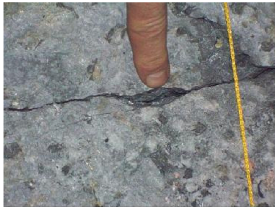
Figure 2. A cooling crack formed in the cathode block after an extended power interruption and cell shutdown.
