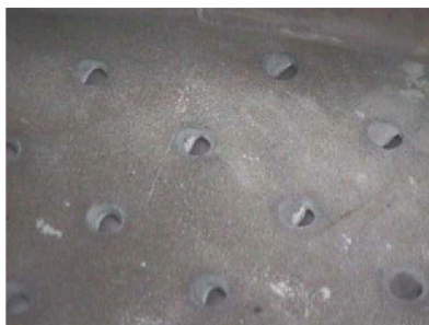
Figure 3 – HGS plugging dribble plates – 2 months after cleaning
