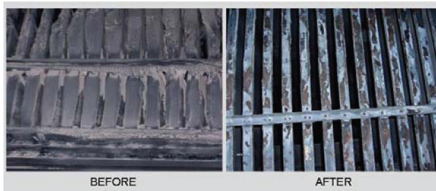
Figure 4 – HGS on diffuser plates before and after cleaning.
