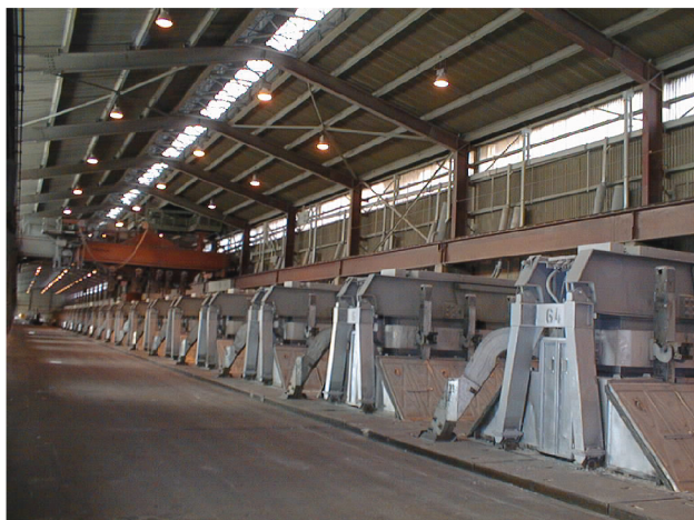
Figure 9: Installed ADS at Hydro Aluminium Karmoy.
