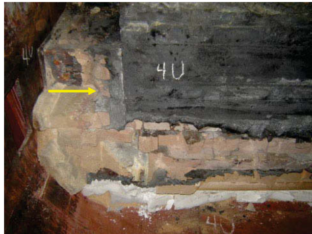
Figure 4. Under-insulated design. Very little bath penetration of refractories as indicated by the arrow
