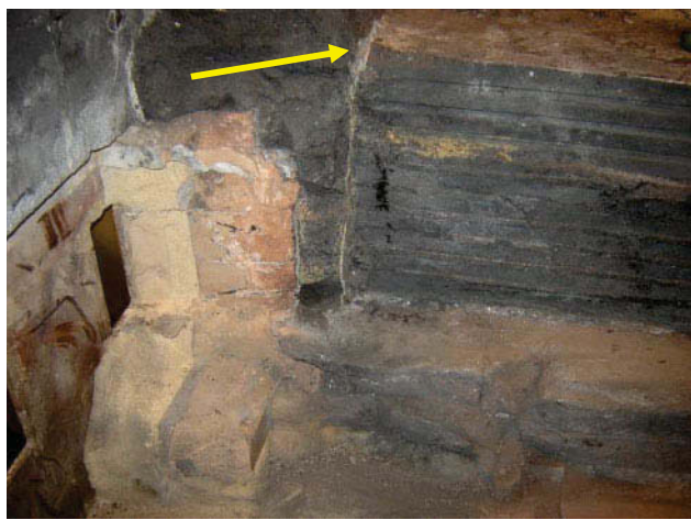
Figure 6: Ramming paste shrinkage in perimeter seam. Age: 28 days.
