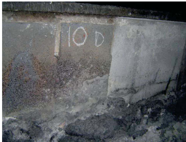
Figure 7. Silicon carbide side-by-side test showing an inferior bonding system on the left
