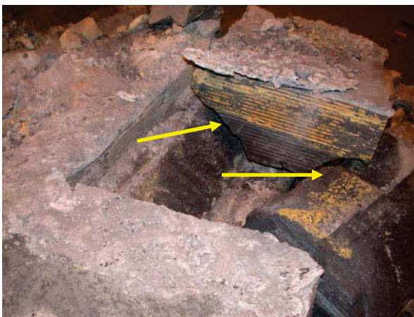
Figure 10: Wing cracks (indicated by arrows) caused by collector bar casting
