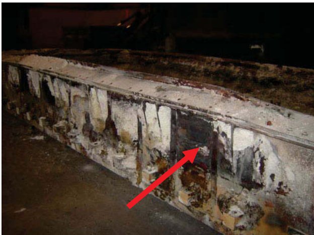
Figure 14: Sidewall failure due to full trenches
