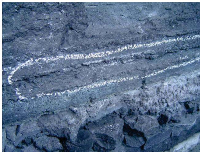
Figure 8: Rammed paste seam with poor bonding between layers seen within chalk marked area.
