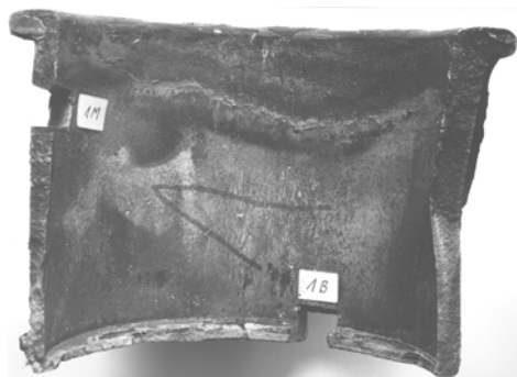
Figure 21: Samples taken from a cast iron thimble for microprobe investigation
