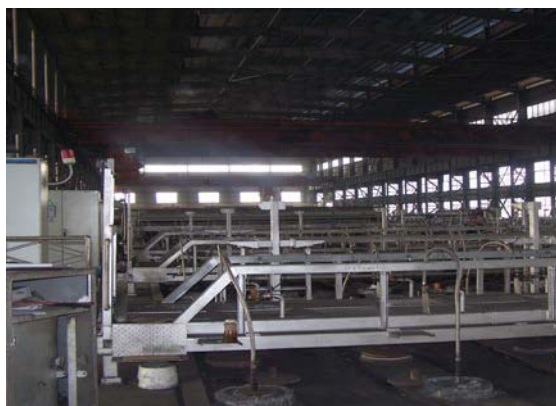
Fig 4 New Firing Control System
