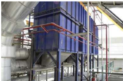
Figure 7: RTO at Qatalum paste plant
