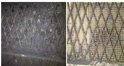
Figure 6: RTO grids before and after a bake-out
