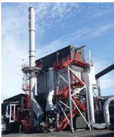
Figure 10: Mosjøen Paste Plant RTO
