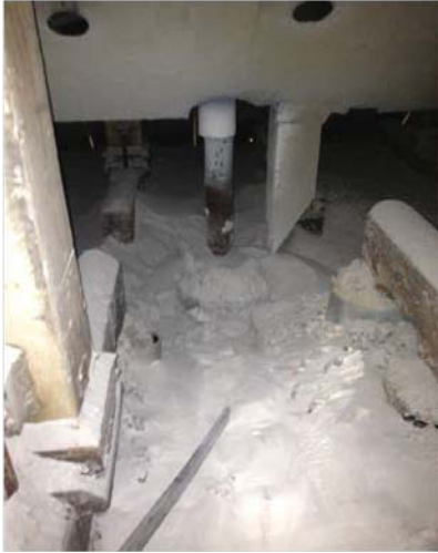
Figure 10. Root Cause of the problem identified – a blocked feeder hole cause by a leaking feeder
