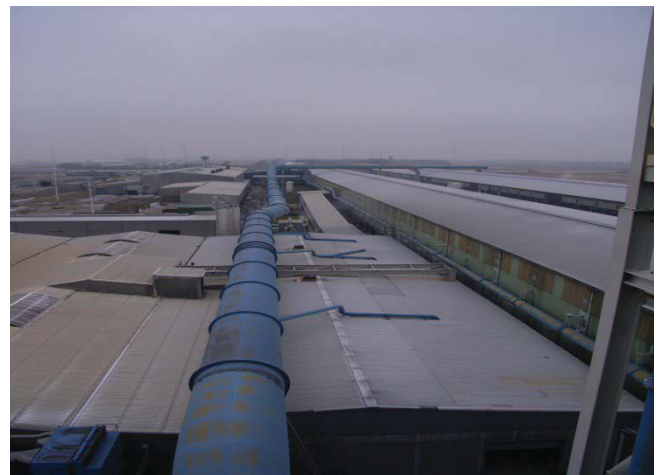
Figure 2: Gas Duct from Potlines to GTC
