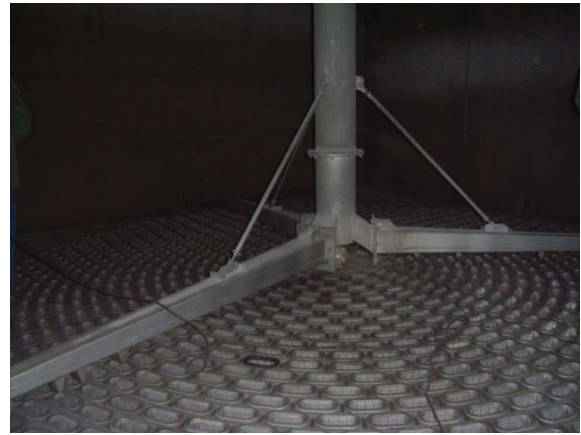
Figure 10: LP Pulse Cleaning System at ALDEL
