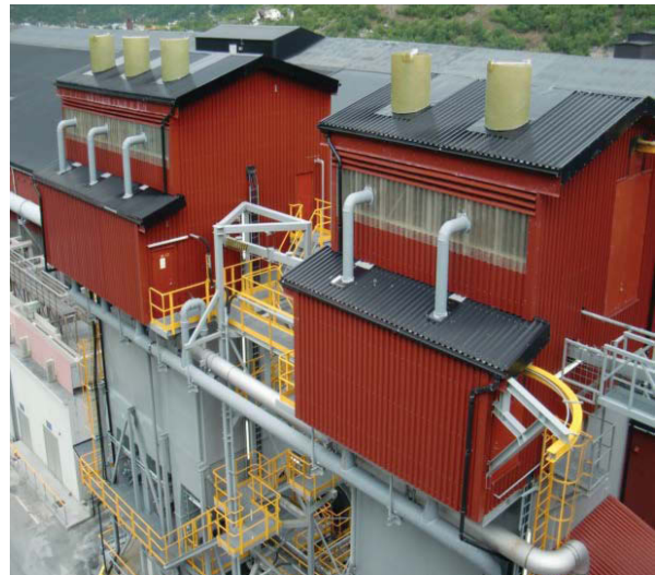
Figure 8. Abart DDS with wet SO 2 scrubbers installed.
