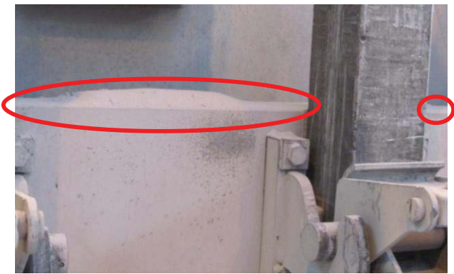
Figure 4. Anode rod clamped in place onto a reduction cell showing stray alumina on top of the anode beam.
