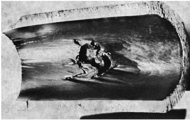
Figure 3: Example 1 of erosion due to high velocity solids flow [2]
