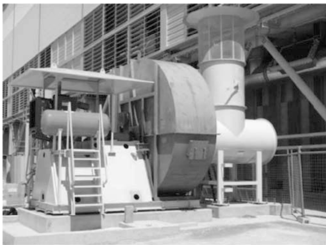
Figure 5. Direct Drive Diesel Powered Emergency Draught Fan
