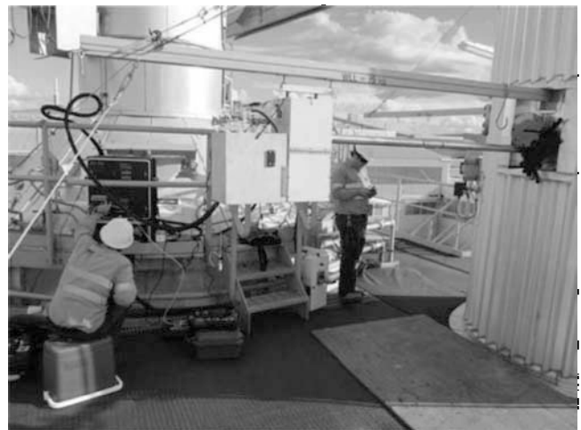
Figure 3. Large Service Platform for Cooling Tower and Exhaust Stack
