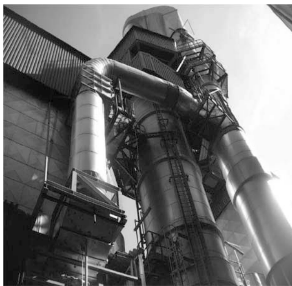
Figure 2: The installed full scale demo AHEx FTC at Alcoa Mosjøen.
