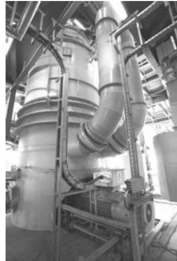
Fig. 4: Vertical Mill for Coke Grinding at EMAL
