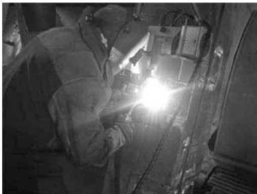
Figure 10 ZeroB in use on a live busbar positive riser
