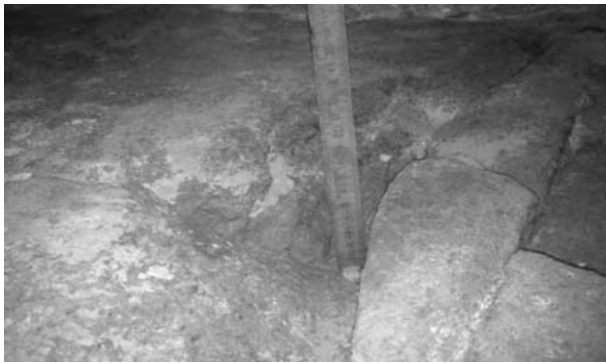
Figure 8. 7 cm lining crack due to metal pad extraction.
