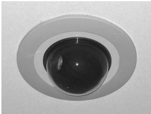
FIGURE 14.2 A ceiling-mounted camera.
